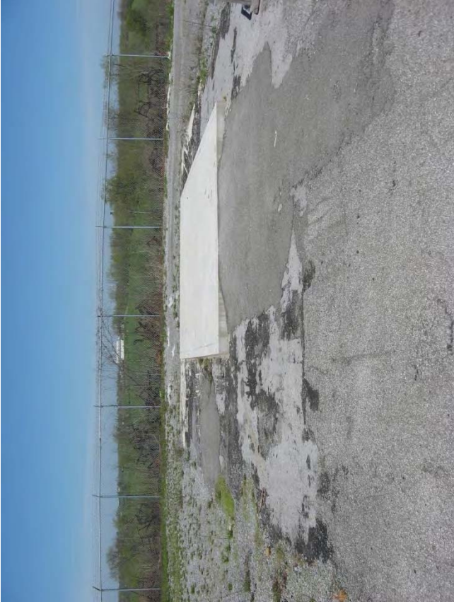
Photo No. 2: Visible staining (B6F-B7F)
